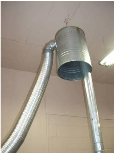
Photo 18: Dilution cap over chimney stove
