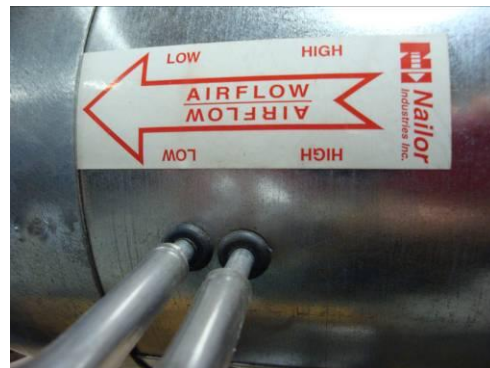
Photo 20: Arrow on flow grid showing direction of flow
